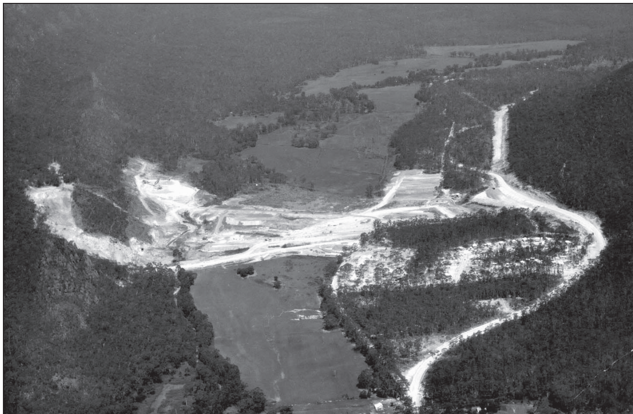
CONSTRUCTION SITE: The first embankment earthworks are undertaken during the construction of the Lake Bellfield reservoir.
